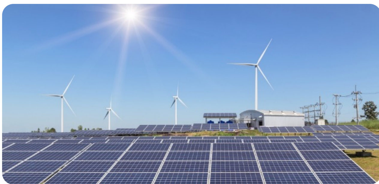
Fig 6- Rows Array Polycrystalline Silicon Solar Panels
